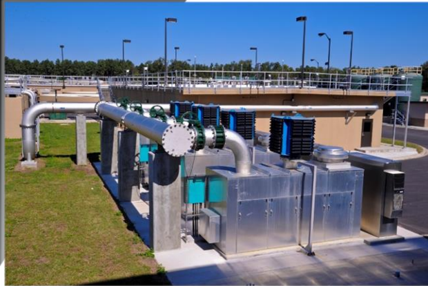
Note: Stainless steel piping is frequently used in water treatment plants because of corrosion resistance and hygienic properties.
